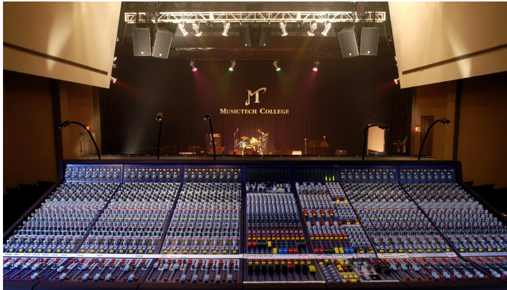
Legend 3000 Mixing Console and Stage with Clusters of Xi Series and Ground-stacked Xi Series Subwoofers
